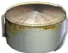
POL storage tank
